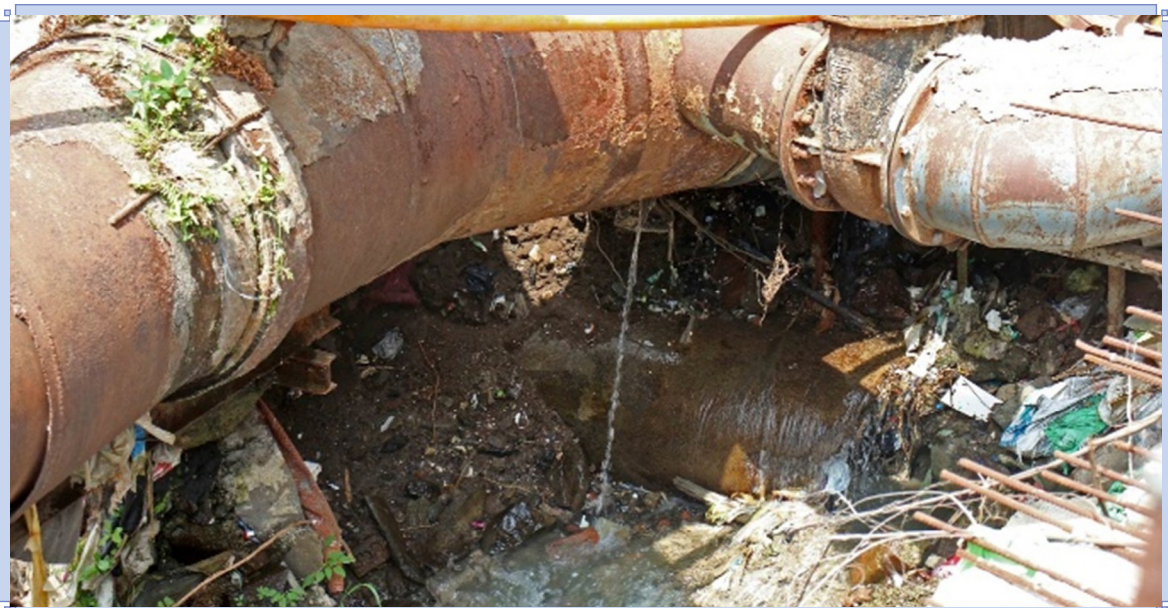
Leaking and corroded water pipelines
