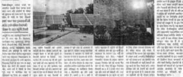
Solar panels installed in Bahrayan village, Mirzapur, showing the use of solar energy for electricity generation.
