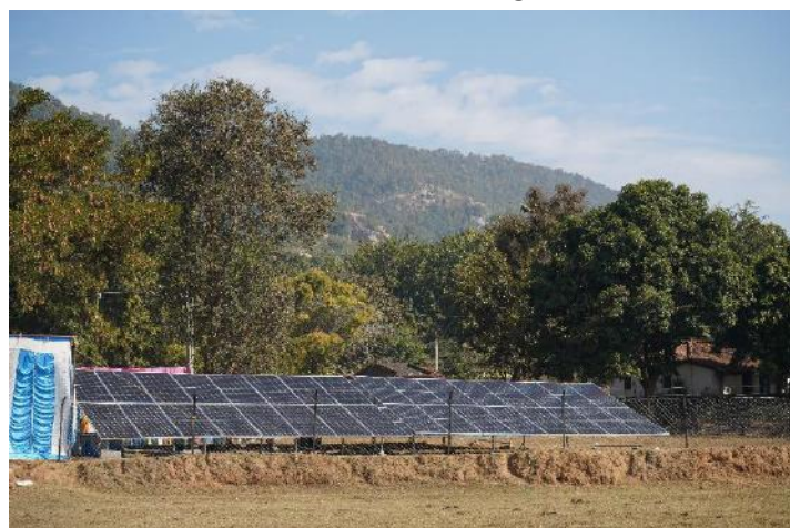
A 32.5 kWp women-led solar mini-grid in Nawagarh Patratoli, Raidih, Gumla district, Jharkhand, providing clean energy and strengthening micro-enterprises for sustainable rural development
