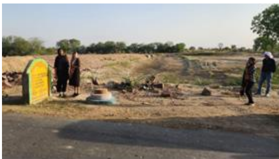
The Development Alternatives team next to an Amrit Sarovar site still under construction in Patharam village
