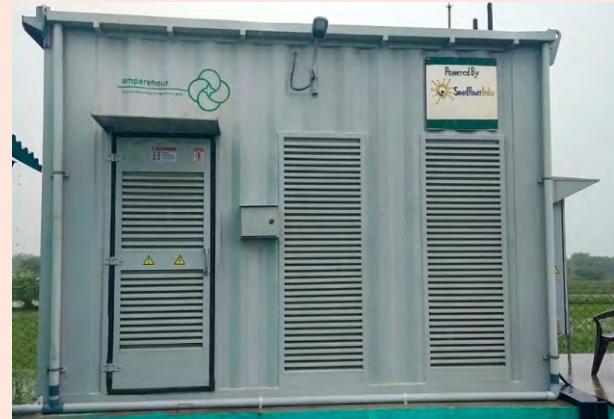
Lithium-ion battery energy storage system and grid-lock, Shivpura, Uttar Pradesh
