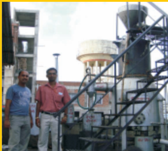
A Rice Husk Power Plant, Bihar
